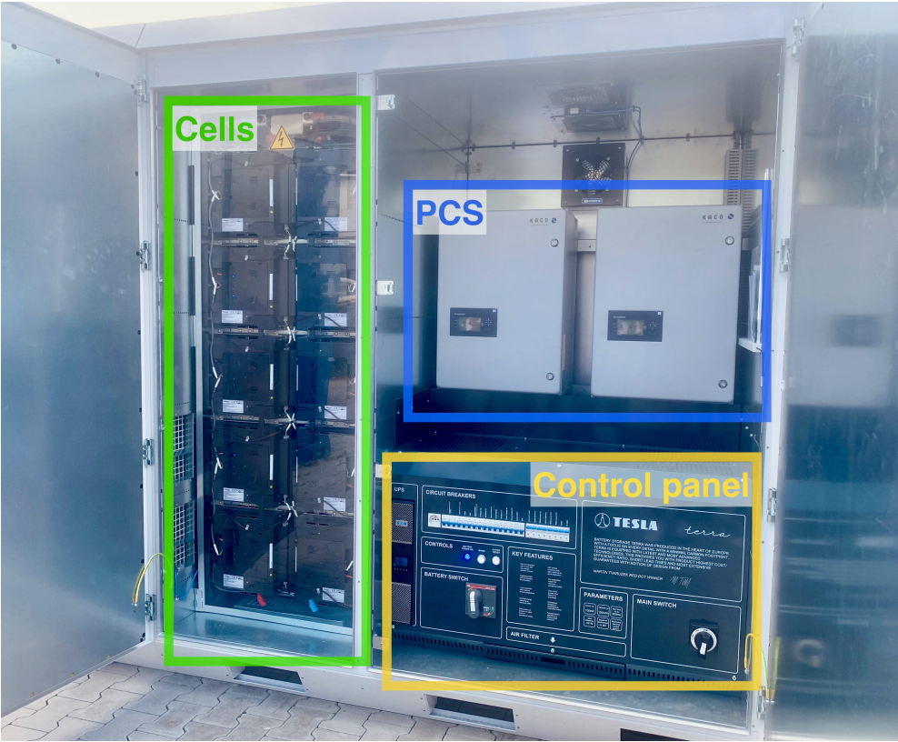
Figure 4.10: Battery container of the 100 kW/151 kWh system. On the left-hand side, battery cells are organized into ten modules; on the right-hand side, the power conversion system (PCS) is located, consisting of two 50 kW inverters and a control panel with the battery management system and switchgear.
