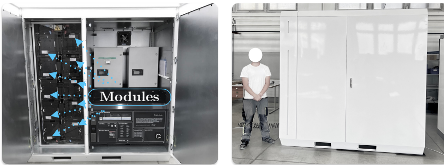
Figure 4.3: The studied TERRA energy storage unit with open doors (left) and closed doors (right). The system has an installed capacity of 151 kWh distributed among 10 modules.
